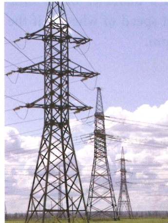
An electricity pylon
